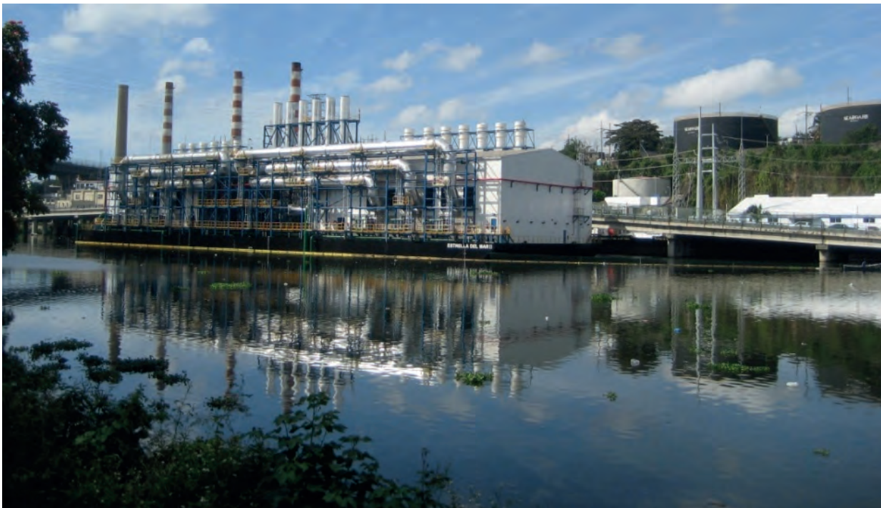
Figure 44: Natural gas fuelled power barge for generation of electricity moored in the city centre of Santa Domingo and supplied by gas from the Andres LNG import terminal and regasification plant
