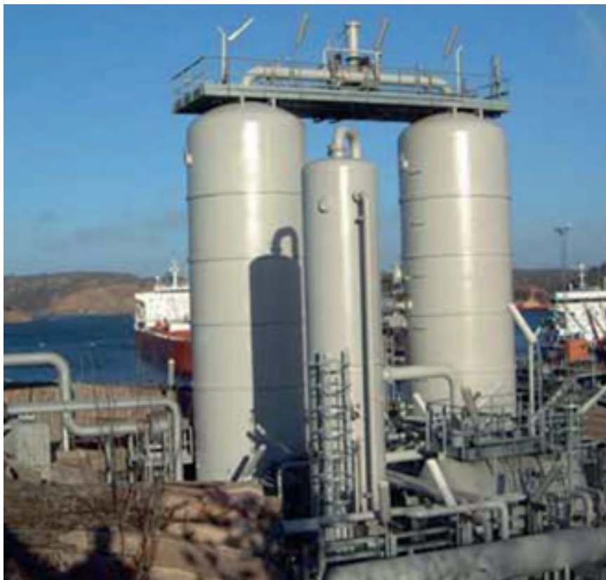
On-shore vapour recovery unit
